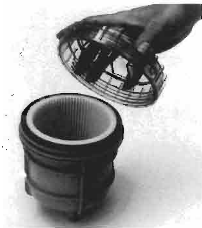
Controle koelwaterfilter. Checking raw water strainer.
